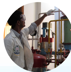
Bio-diesel plant 50 L Capacity
